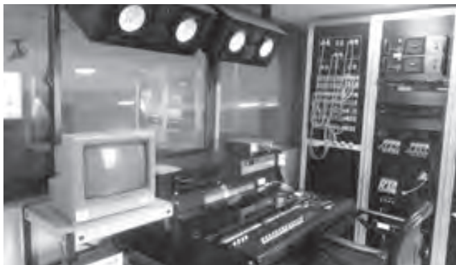
劣化が進む機材
